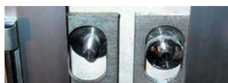
Coupling joint in shaft-box facade (above); fixing brackets at slab edges (below)
