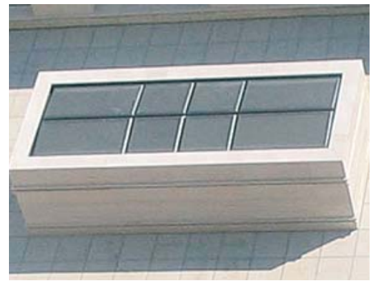
Smoke vent housing
