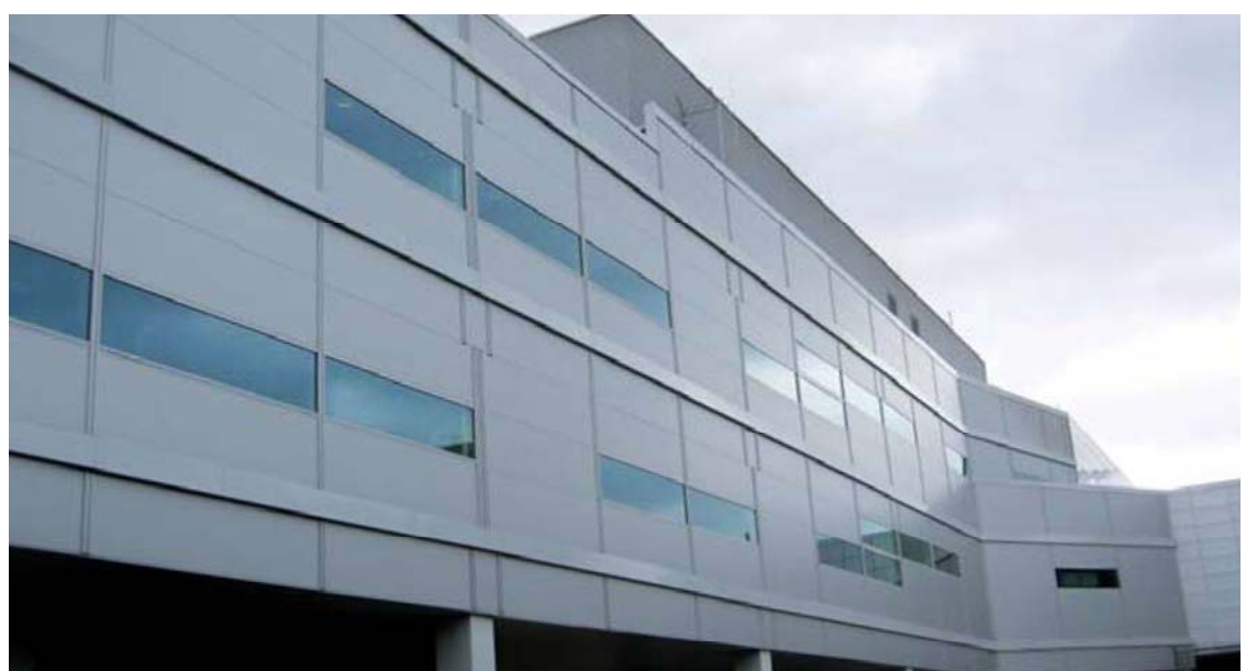
Passageway link with fire-rated curtain wall
